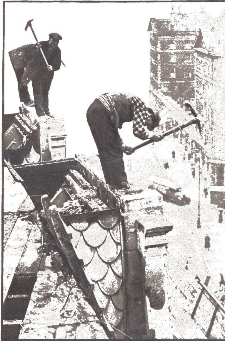
"Like cats, they climb, and only require a foothold on the edge of a precipice to work comfortably . . . most would scorn any class of building work."
