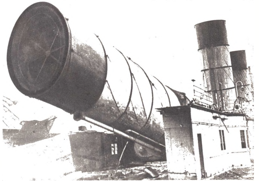
Down comes one of the Mauretania's mighty funnels in the ship-breaker's yard. But the metal will be used again.
